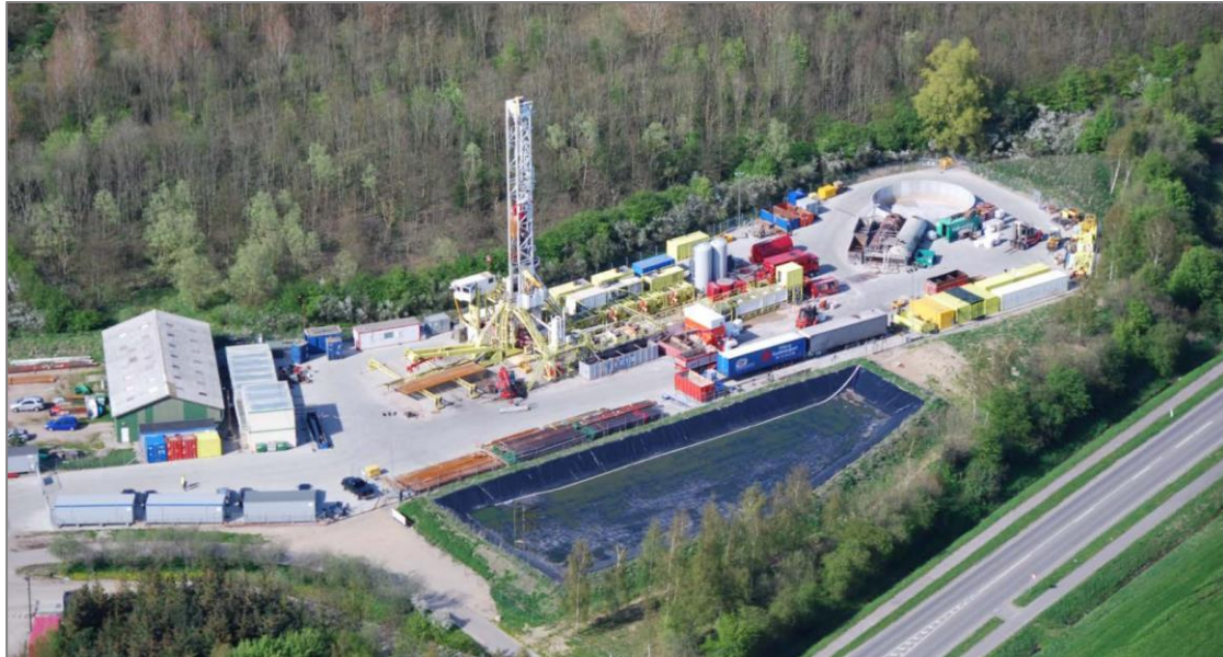
A borehole drilled in Denmark to supply hot water to a district heating scheme (source: www.geotermi.dk )
